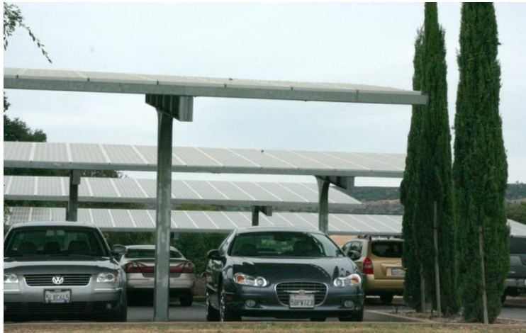
Solar panels on structures covering surface parking lot
