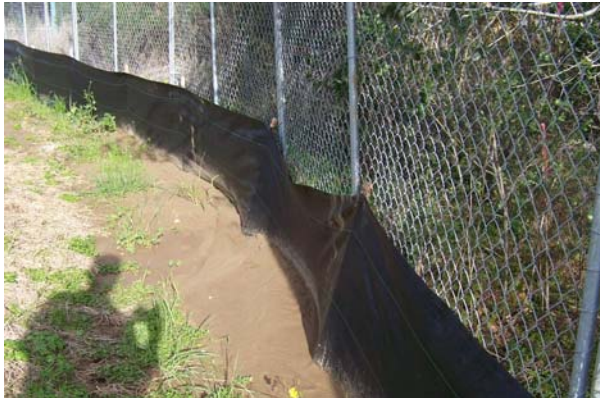
Picture 10. Silt fencing that needs a little bit of maintenance.
