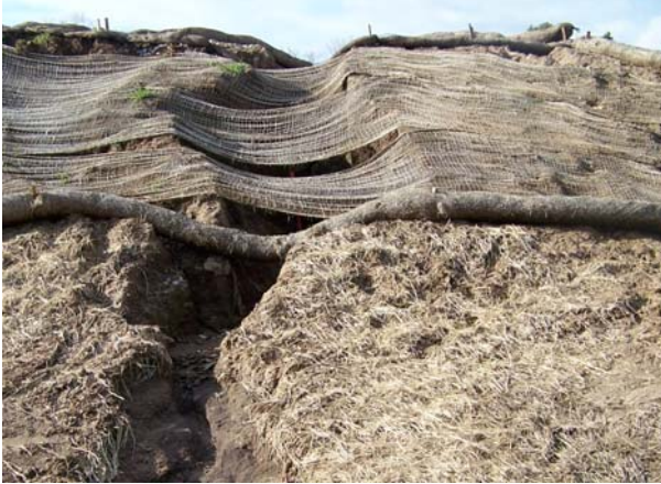
Picture 7. Result of concentrated water flowing over a fill slope.
