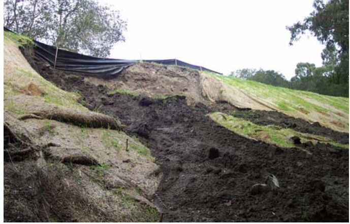
Picture 8. Result of concentrated water flowing over a fill slope.
