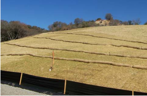
Picture 4. Use of straw rolls on a slope with a silt fence at the bottom of the slope. Note: This slope has also been seeded, and the steeper portions have been covered with erosion control blankets.
