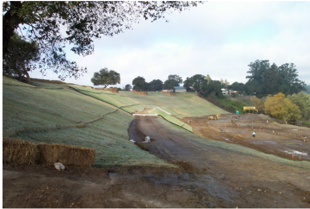
Picture 2. Effective use of erosion control blankets placed on a steep slope. Seed was spread prior to placing the blankets.
