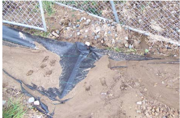
Picture 11. Silt fencing that needs a lot of maintenance.
